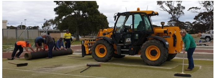
Dunn Rock Tennis Club hard at work removing the artificial lawn at the Lake Grace Tennis Courts.
