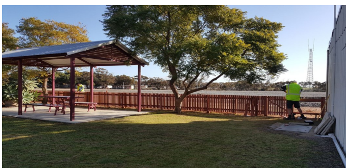
Above: The new fence to prevent access to the railway line, creating a safe picnic area.
