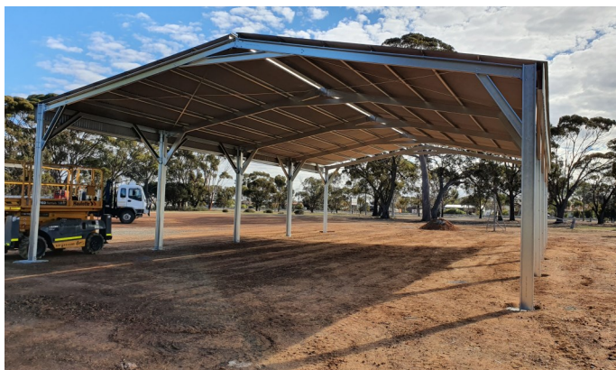
Above: Shade shelter ready for jumping pillow to be installed in Lake Grace
