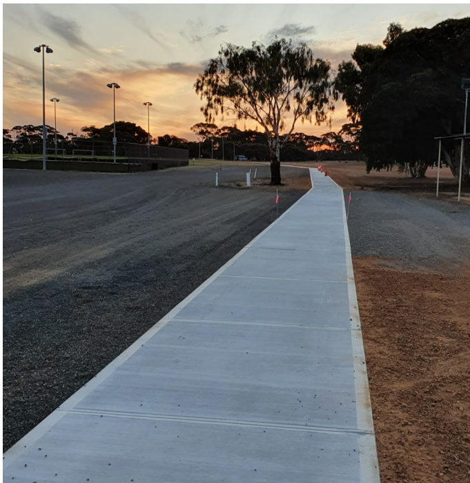
The new footpath going through the Lake Grace recreation grounds from the entrance to the medical centre was completed.
