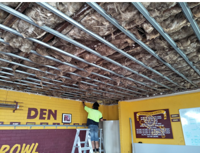
Above: Hue replacing ceiling battens in the change room at Newdegate Pavilion
