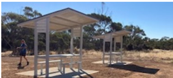
The installation of 2 new shelters at the Newdegate Silo art viewing area.
